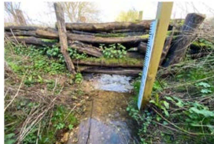
Old style leaky dam still functioning after seven years
