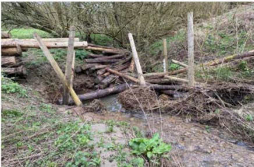
Dam collapsed catastrophically. All logs trapped trees and a narrow channel
