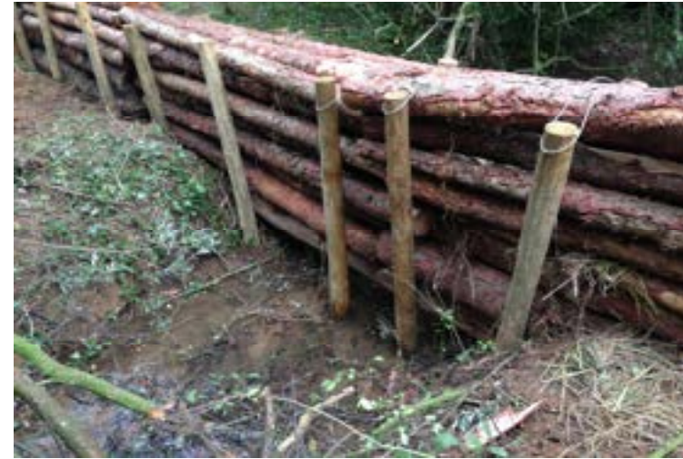
Old style leaky dam as built
