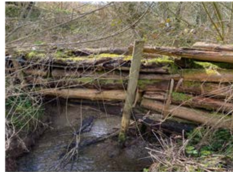
Seven year-old dam, still functioning but with some rotting timbers
