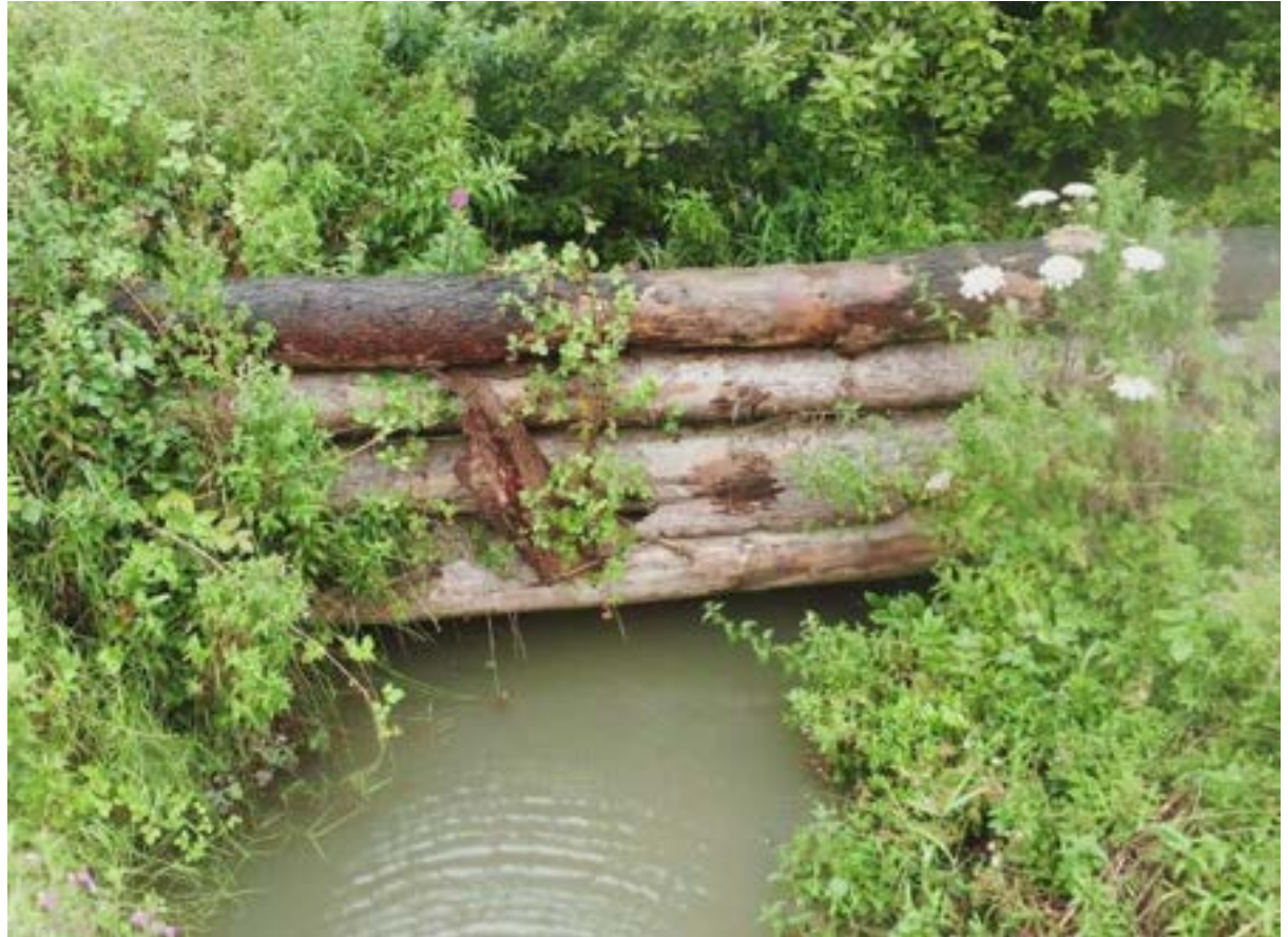
Leaky dam on the Eye Brook
