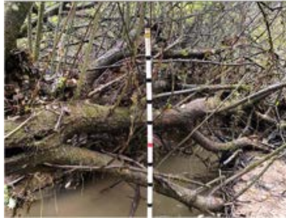
Hinged willow: stable and apparently effective after 2023/24 flooding that caused catastrophic loss of an adjacent traditional dam
