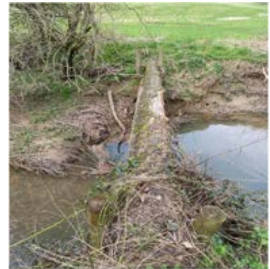
Significant bank erosion around a new style dam following 2023/24 flood events
