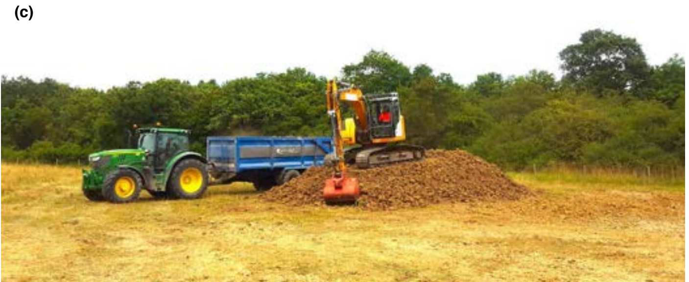
(c) Medium sized ponds of 200-500 m 2 can be excavated using 15 tonne machines. Larger ponds are more efficiently created with larger machines.
